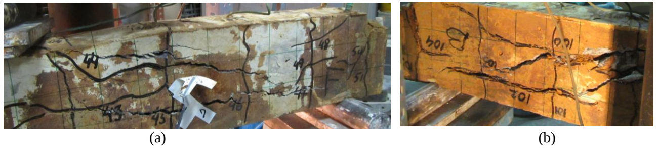
Figure 3.42 Formation of shear cracks during bending test of B24S-FS-13/120
