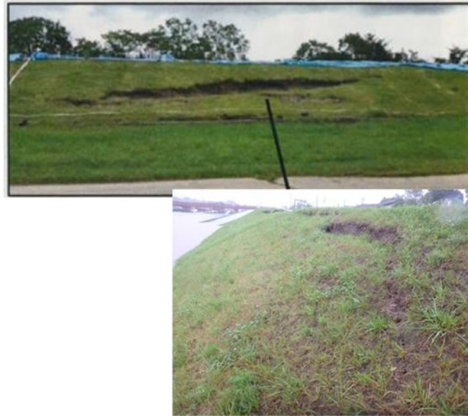
Figure 2.2. Photographs showing shallow slope failure in Kushiro River dyke due to heavy rainfall in August 2016 (Source: Final investigation report Japanese Geotechnical Society Hokkaido Branch)
