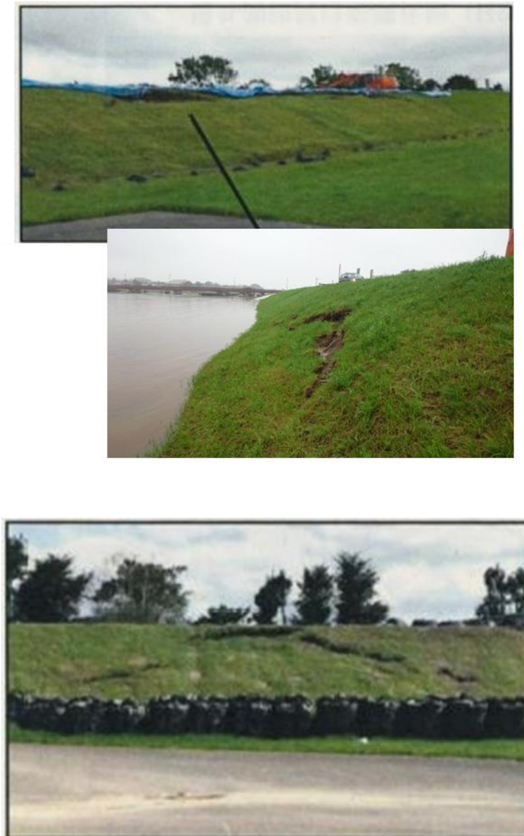
Figure 3.1. Photographs showing shallow slope failure in Kushi River dyke due to heavy rainfall in August 2016 (Source: Final investigation report by the Japanese Geotechnical Society Hokkaido Branch)
