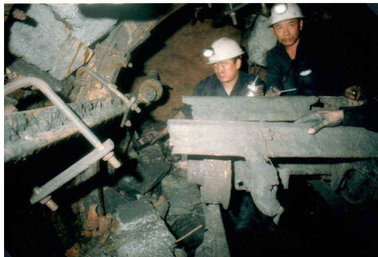
Figure 2-5: Narrowing the return gate roadway due to floor heave at Hong Thai Coal Mine
