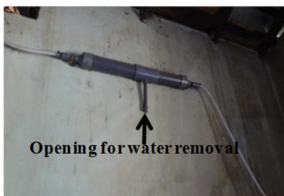
Figure 3- 5 Manual condensed water removal traps
