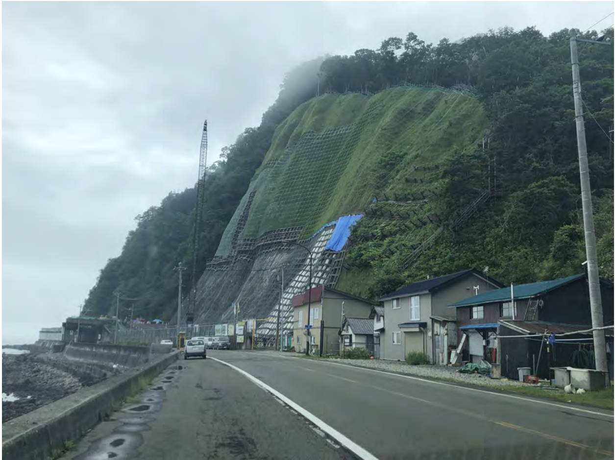
Figure 12: Aftermath of the Ogon Road landslide (photo taken in 2018).
