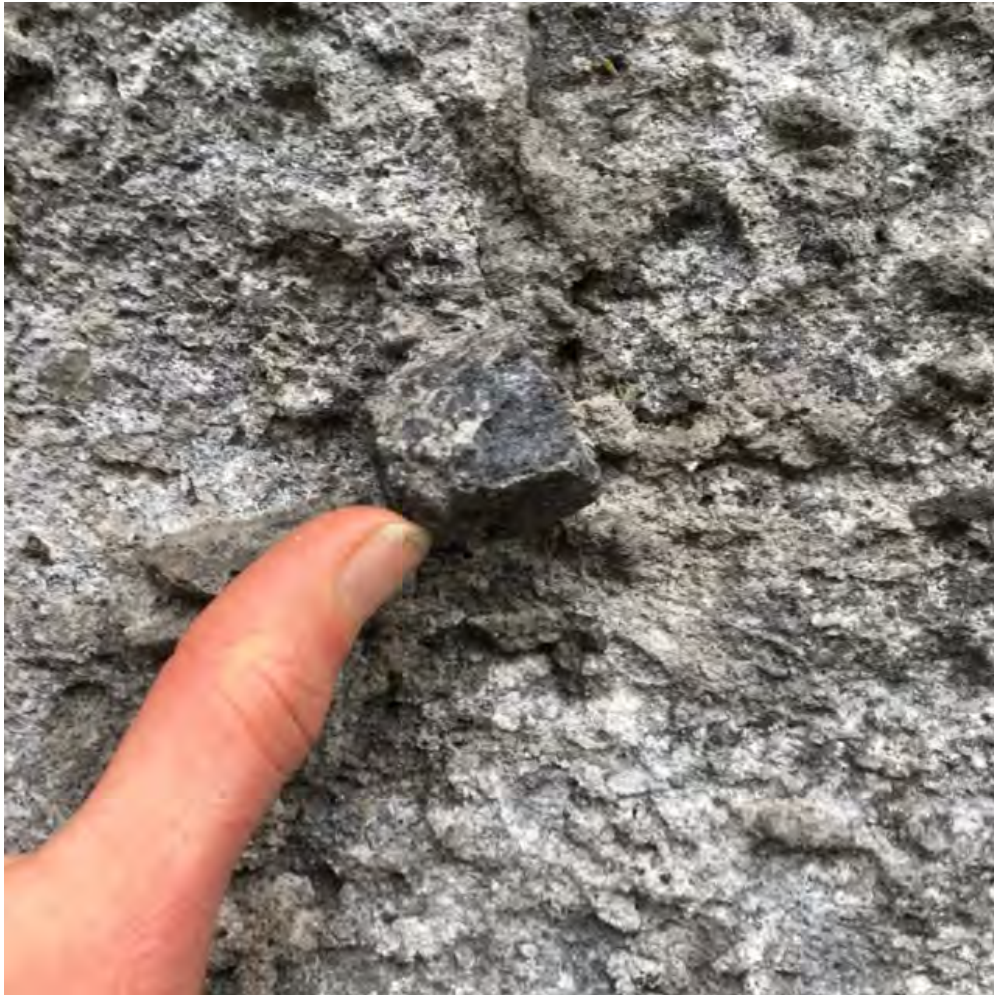
Figure 45: An example of the angular, dark grey fragments protruding from the wall of the tuff cliffs.
