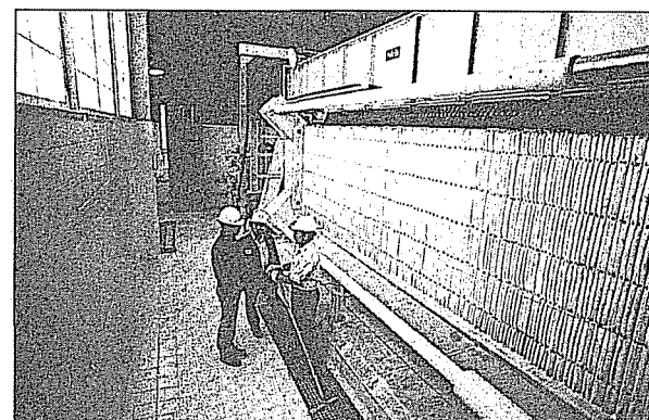
Sludge dewatering filter press
