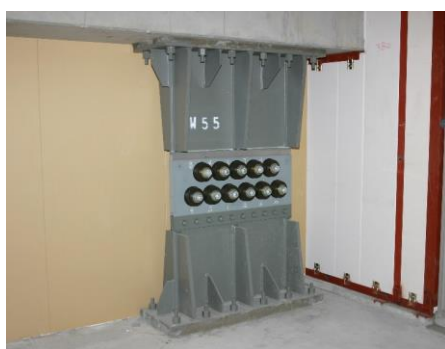
Fig. 2.2.2 Example of the developed stud-type damper with multiple friction units (total sliding force of 1100 kN) installed in an actual building 2)
