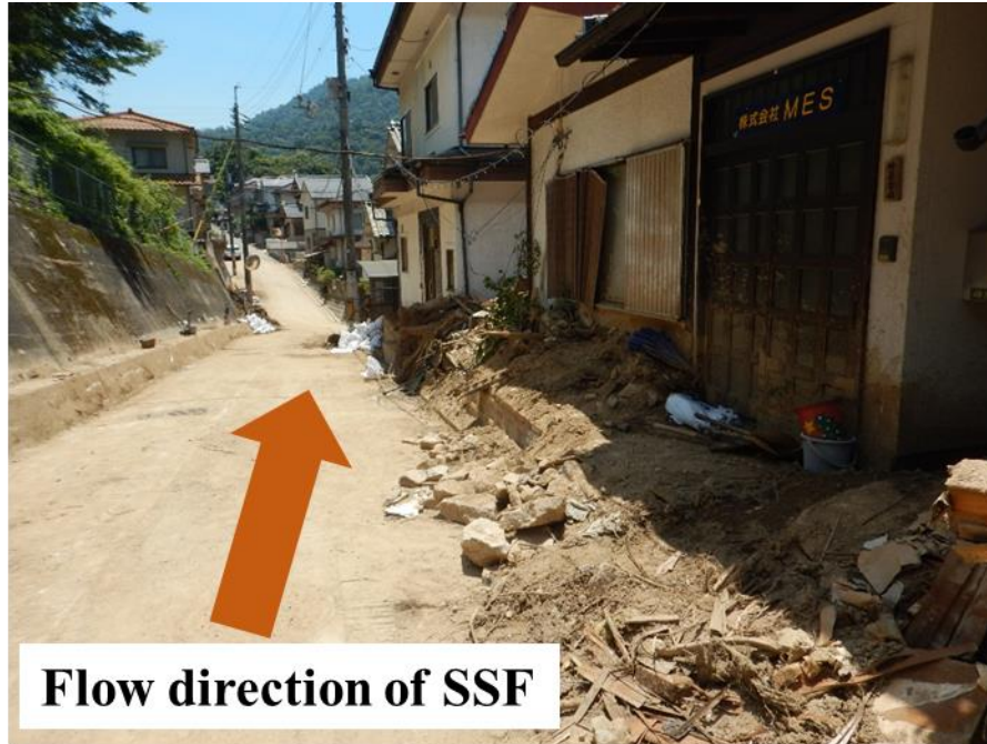
Fig. 1-4. Trace of damage from SSF
