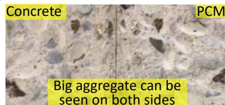
(c) Cohesive concrete failure after cooling
