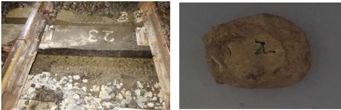
Figure 3-5 Aged ballast particle extracted from the actual ballasted track: (a) ballast particle in the track; (b) a typical ballast particle.
