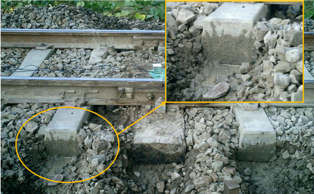
Figure 1-2 Fouled ballast in the aged existing line.
