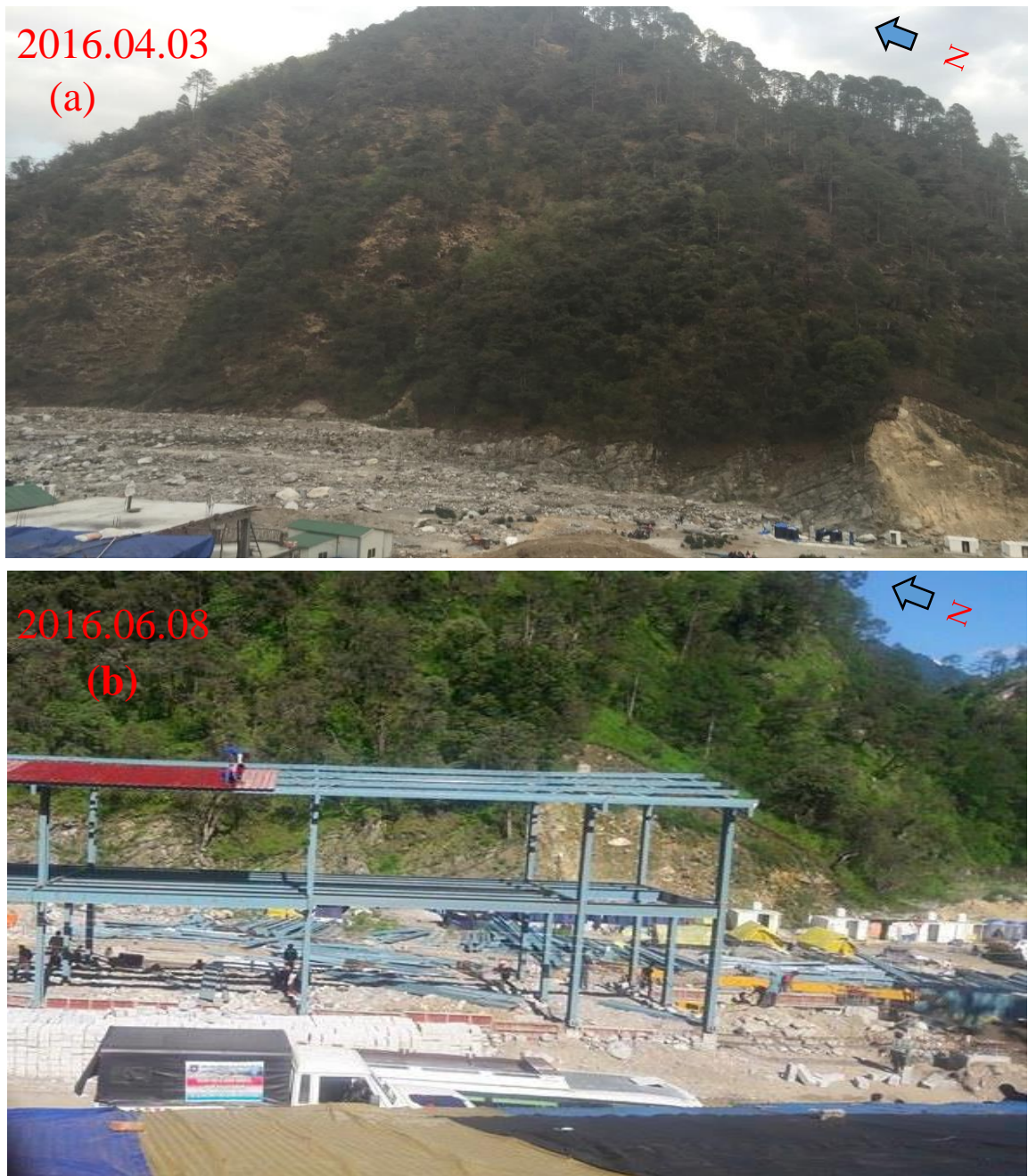
Figure 7.3. An example of re-development of infrastructure for tourism activities at Sonprayag, Rudraprayag district. (a) field photo after the damages of infrastructure, and (b) re-infrastructure for tourism activities (Photo: Amit Kumar Batar)
