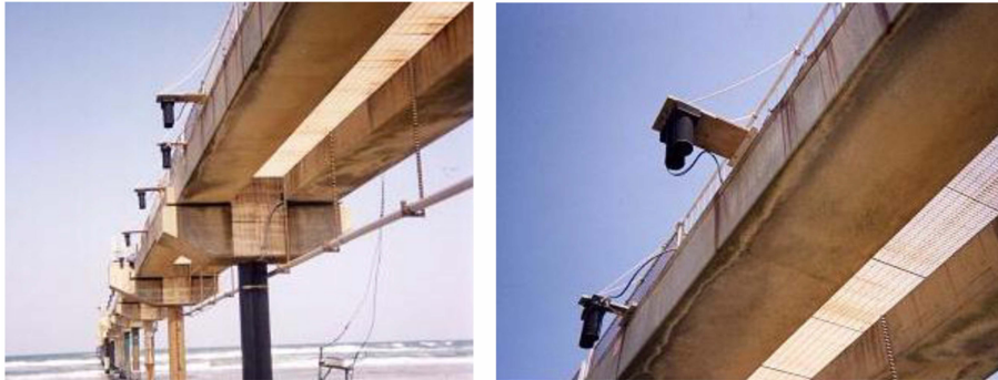
図 1.10 Wave gauges installed along the pier and their close-up view, Mizuguchi (2010)
