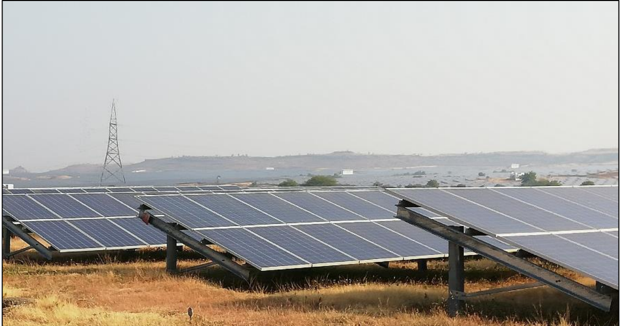
(a) 80MW Avaada Solar power plant, Chalisgaon, Maharashtra
