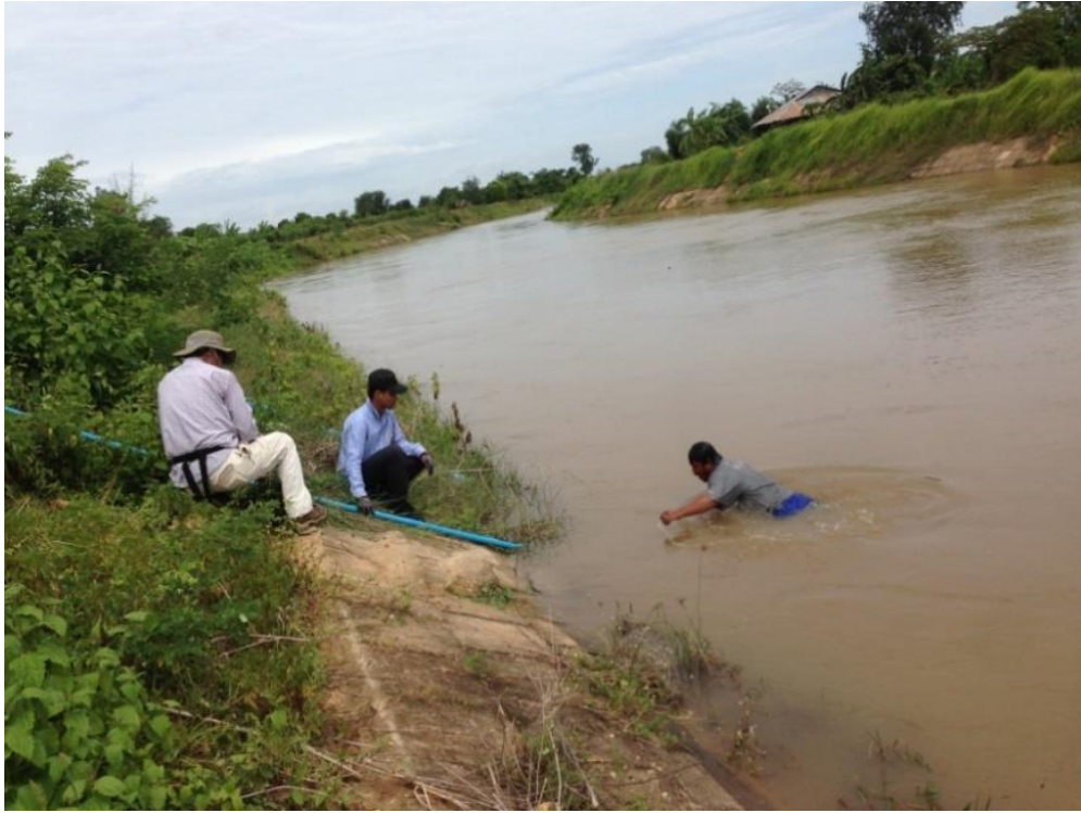
Figure 4-8 Installation of water level logger at the right main canal
