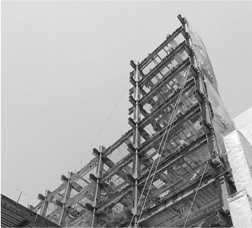
Figure 1.1 A steel moment-resisting frame recently built in Sapporo, Japan
