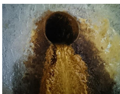
(a) Accumulation of fines around drainage pipe outlet
