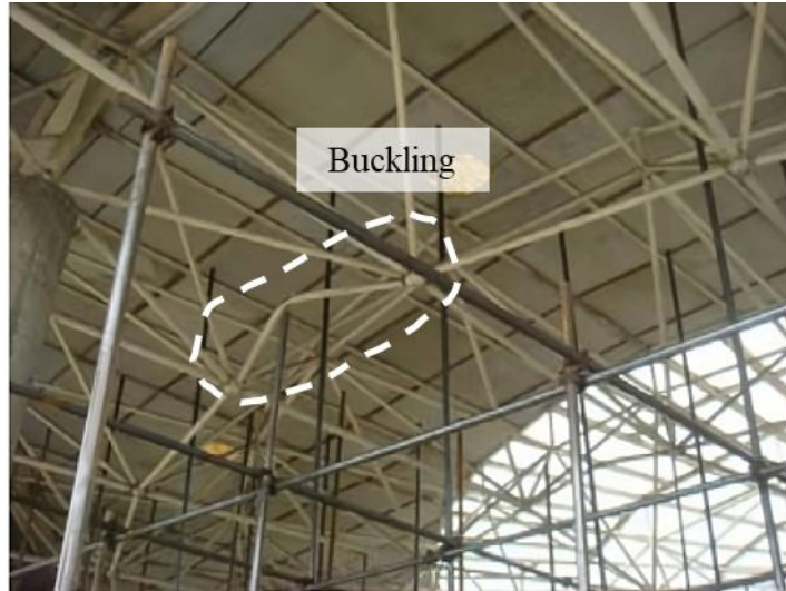
Figure 2.3 Buckling of a member observed in a grid shell located in Mianyang City after the Wenchuan Earthquake (2008) (source: IASS WG8 2019)
