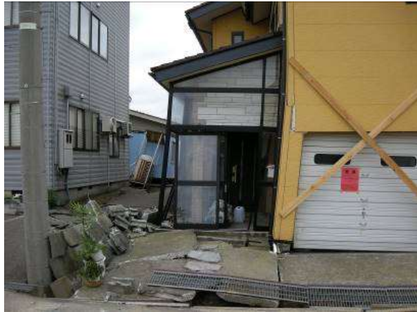
(a) the severest damaged house
