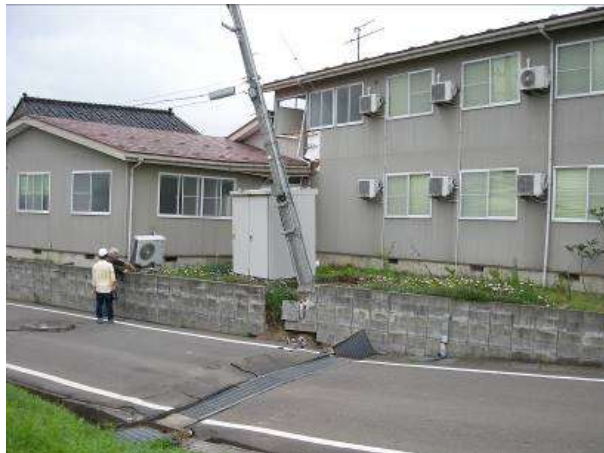
(b) damaged houses due to ground crack
