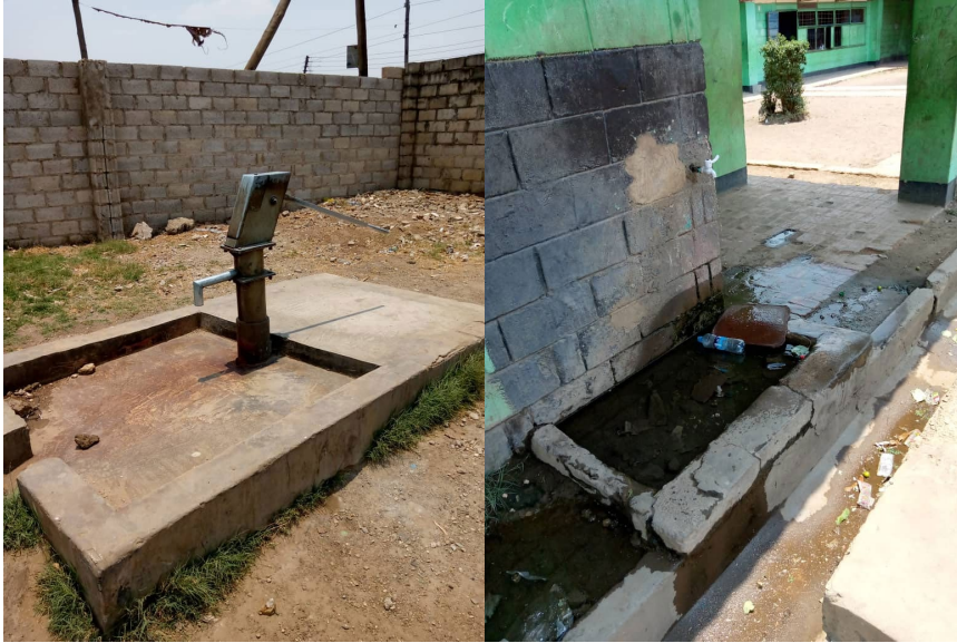
Figure 1 | School mono-pump and unsanitary handwashing tap.
