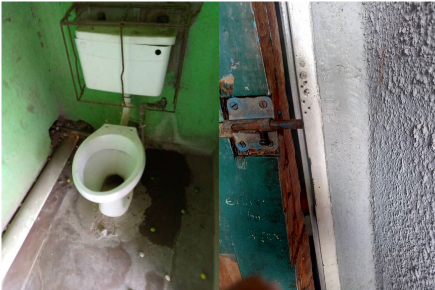
Figure 2 | Schoolgirls' toilets in unsanitary and unhygienic conditions.
